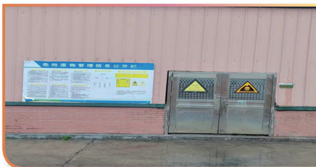
Standardized management of hazardous waste warehouses 危廢倉庫標準化管理
