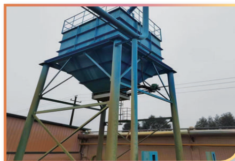
Centralized sludge recycling at sewage stations 污水站污泥集中回收
