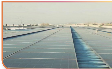
Ma'anshan company installed 1.8MW of new photovoltaic energy 達利馬鞍山公司安裝 1.8 兆瓦光伏新能源
